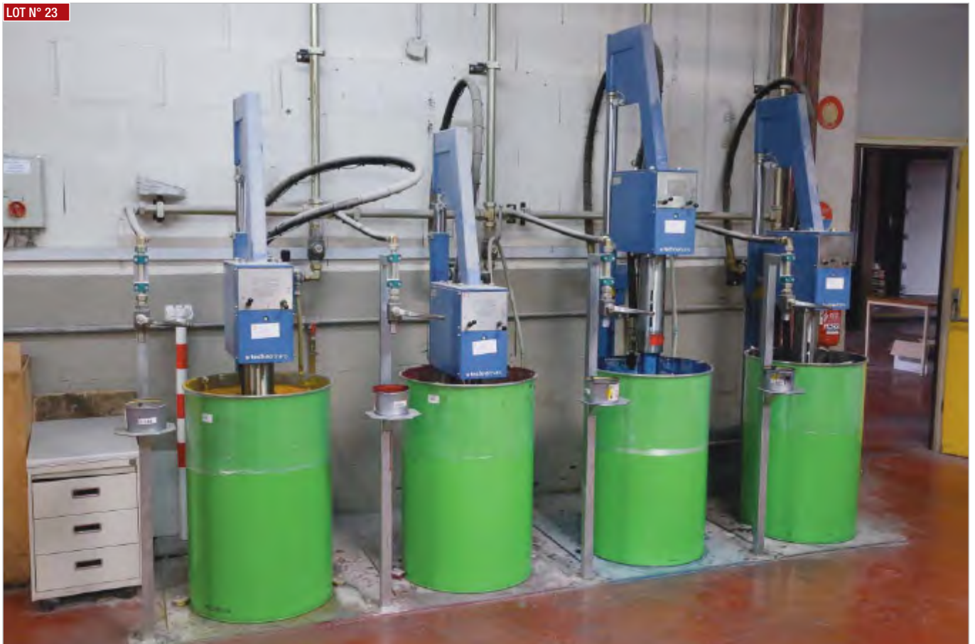
► Installation de distribution des encres comprenant 4 groupes pompe TECHNOTRANS, mod TPB200-36/12 ► Ink distribution device including: 4 TECHNOTRANS pumps, type TBP200-36/12, year 2003
